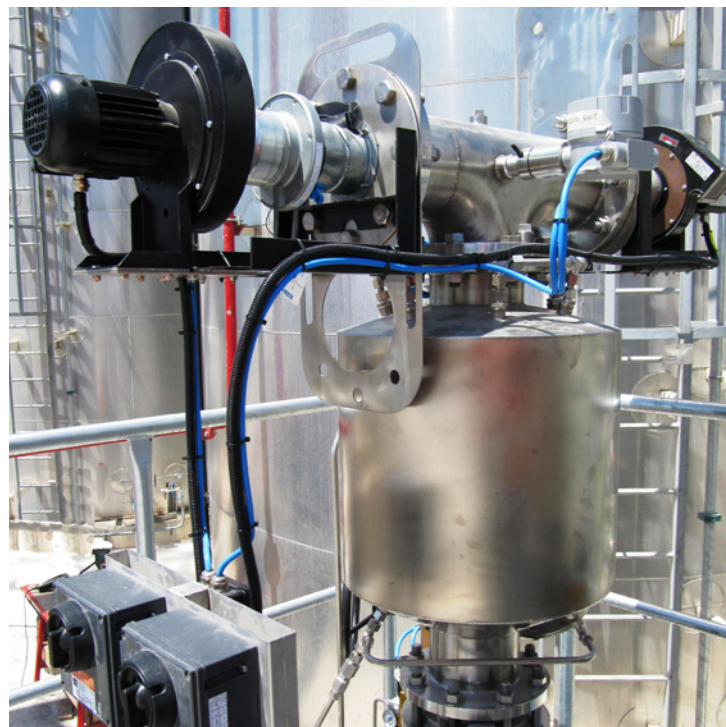
Tank Vent Odour Filter with Automatic Shut-off Valve, Emergency Water Mist System and a redundant Forced Ventilation System.
